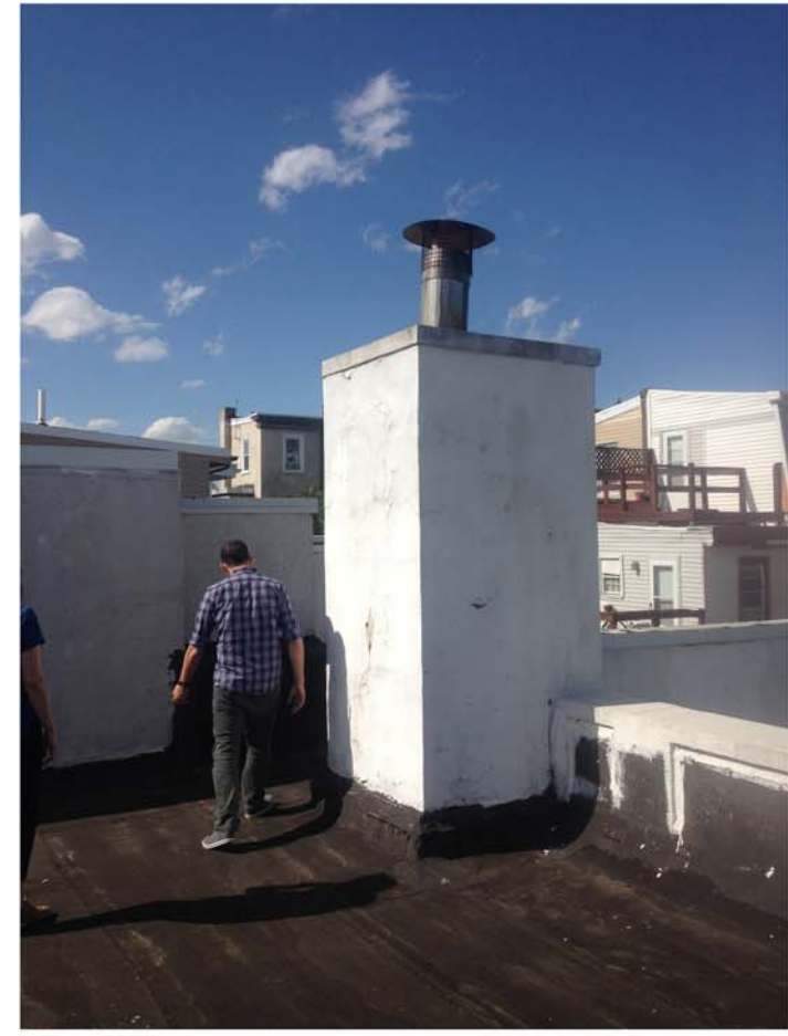
Pictured here is the chase that houses the water lines that service the bathroom below, and vents the boiler through the roof.
